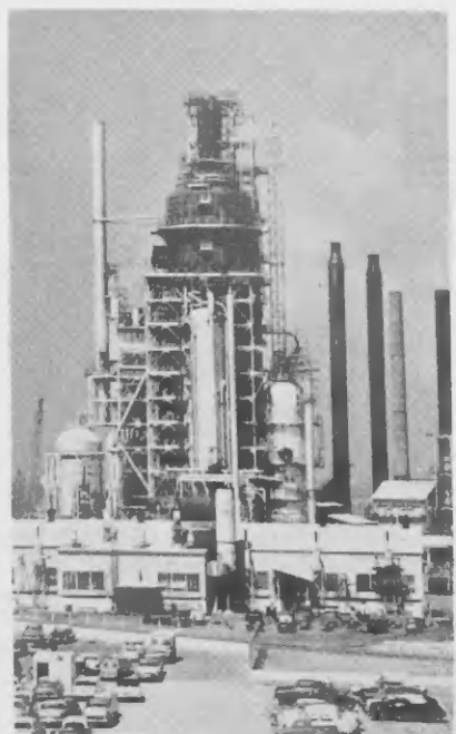
A MAJOR operation at Lago is the Cat Cracker turnaround. See pages 4 and 5 for turnaround men at work.
